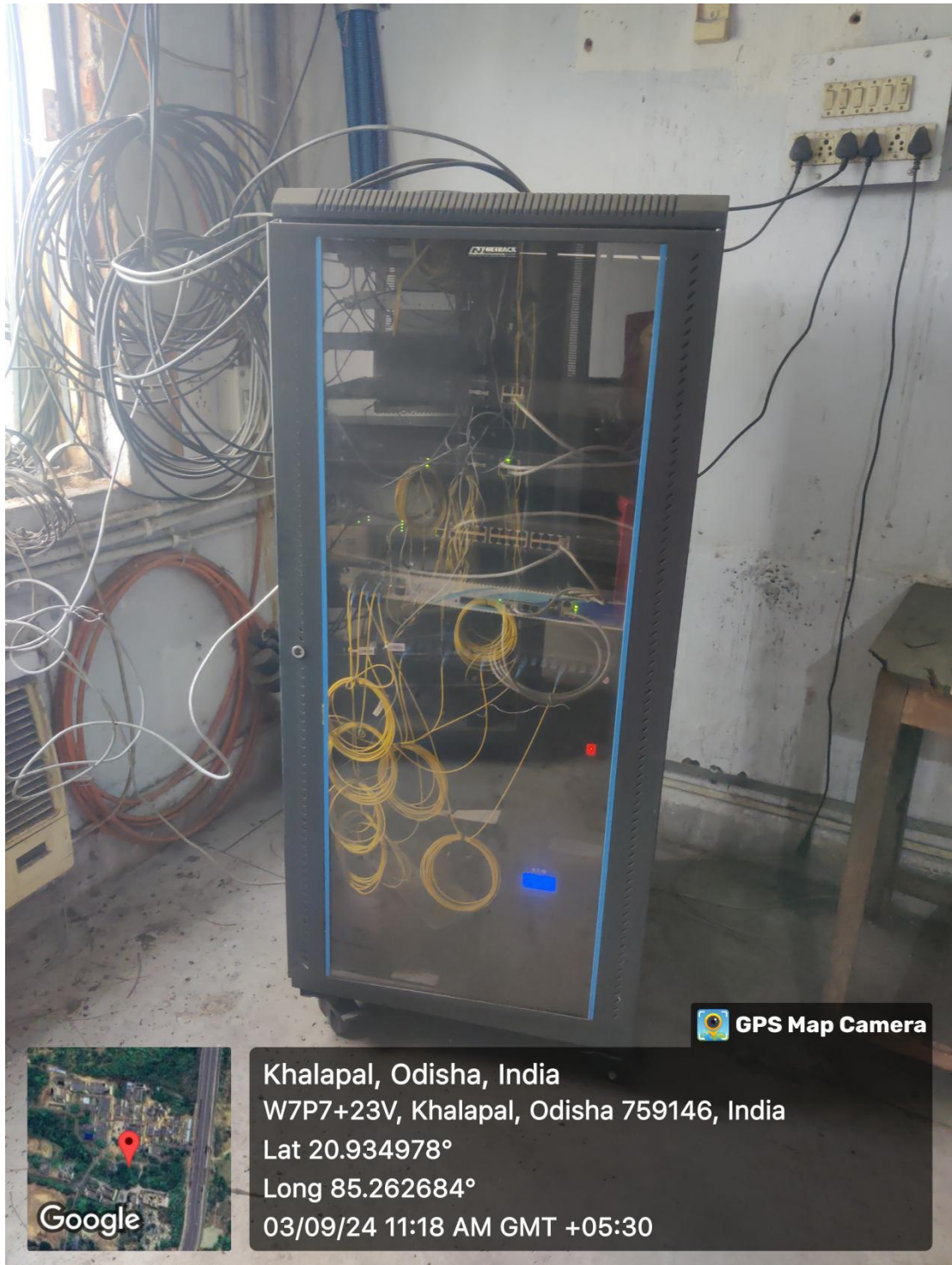
SERVER ROOM (OLD ACADEMIC BUILDING)
