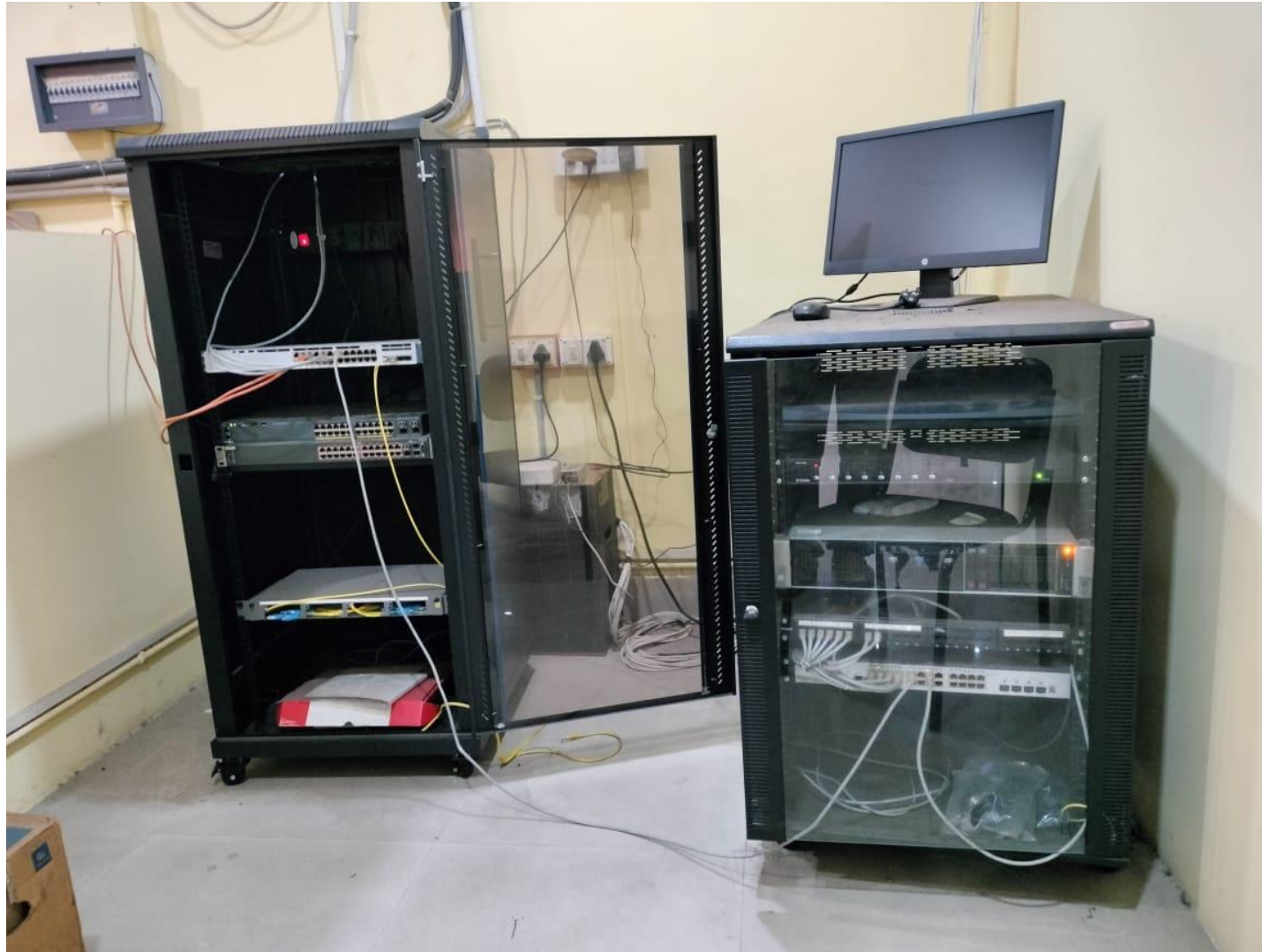
SERVER ROOM (NEW ACADEMIC BUILDING)
